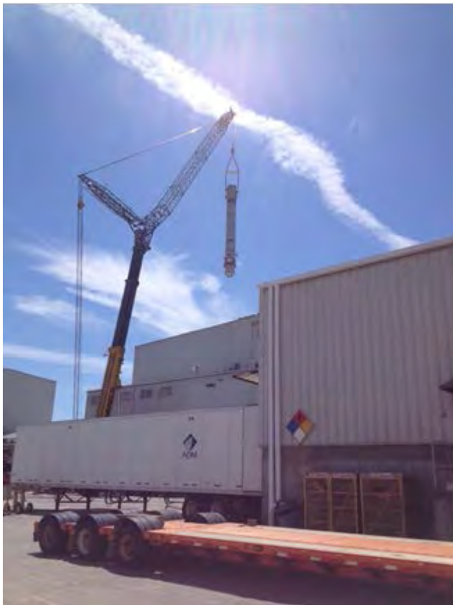
Figure 9 Evaporator installation for East Plant Soy Molasses Removal
